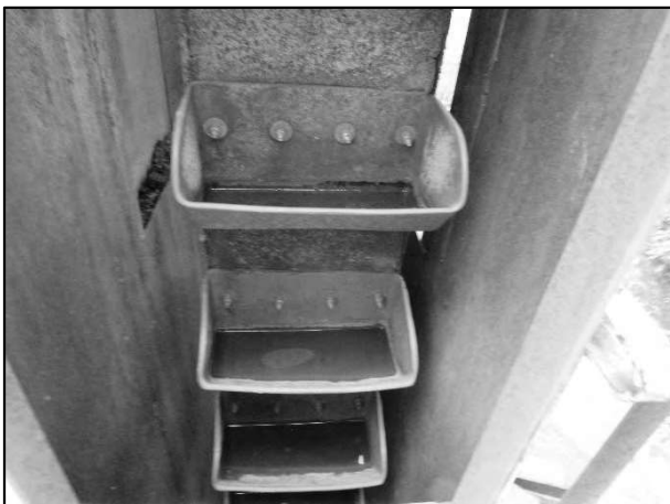
7M – Feed Mill Legs / Water Damage – No Value
